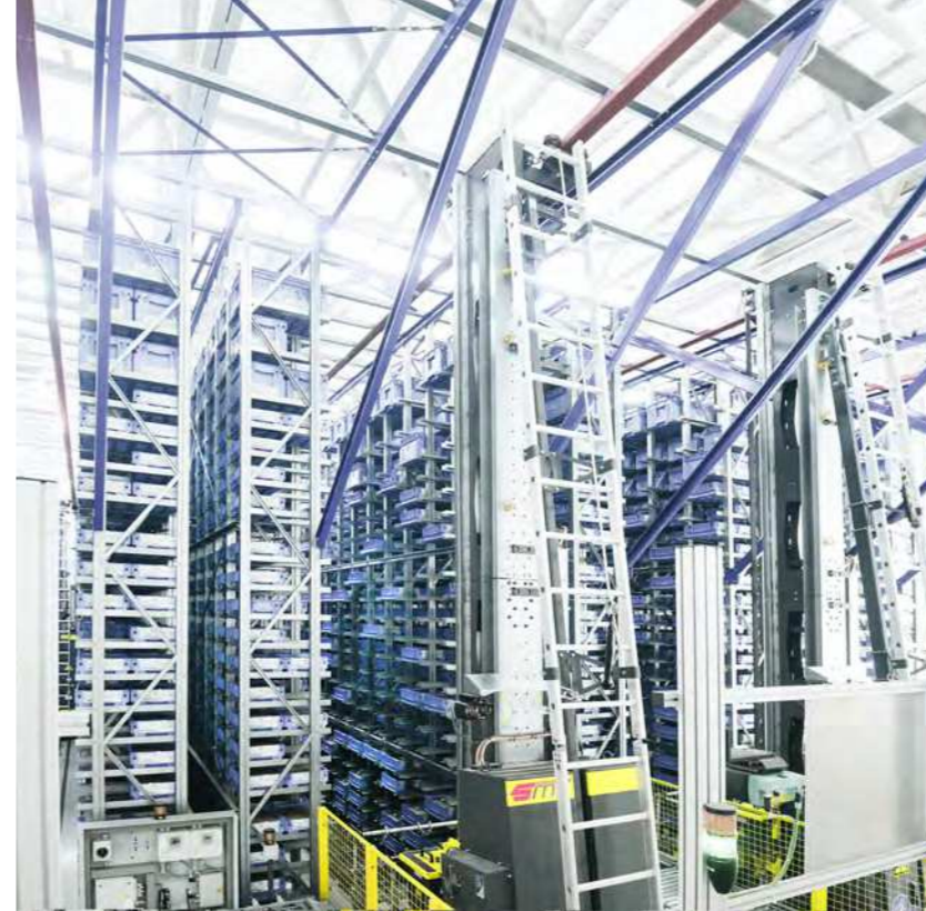
SSI Miniload Automated Storage and Retrieval System (ASRS)
