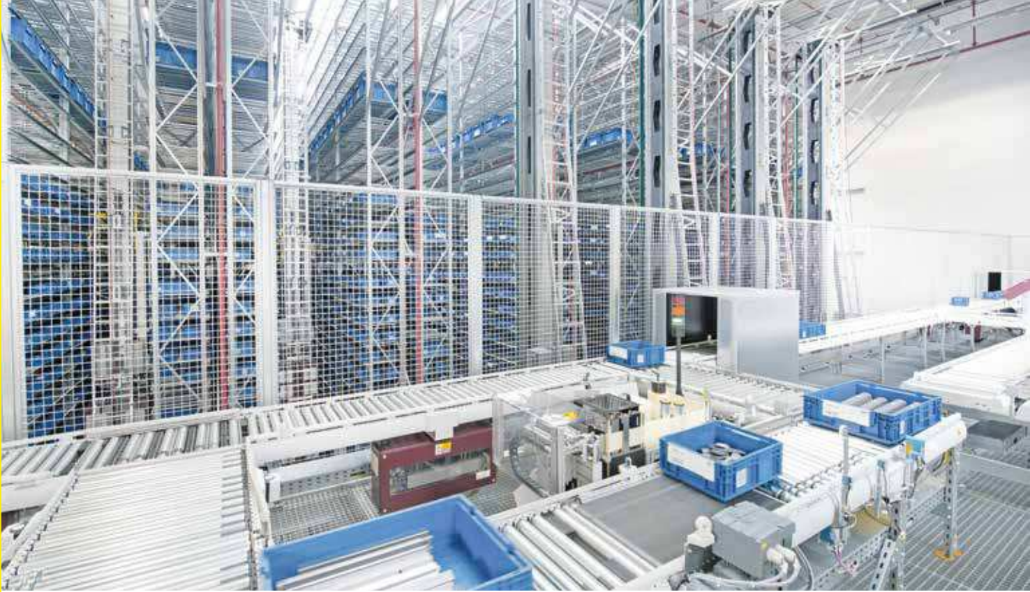
The seven Schäfer Miniload Cranes generate a turnover of 840 bins an hour.
