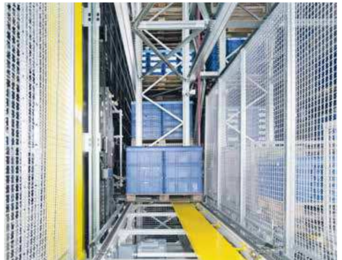
The high-bay warehouse acts as a replenishment buffer, connected to an existing structure via a bridge construction.
